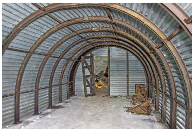
Inside one of the secure stores and looking out to the main repository chamber. The construction method is very similar to the Royal Engineers-built gun shelters of Dover and elsewhere
